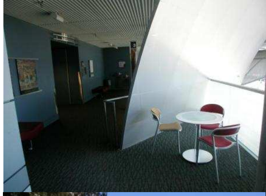
Figure 30 - Panel & Railing on Level 3 are not Cane Detectable
