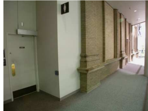
Figure 25 - Protruding Trim at North Atrium
