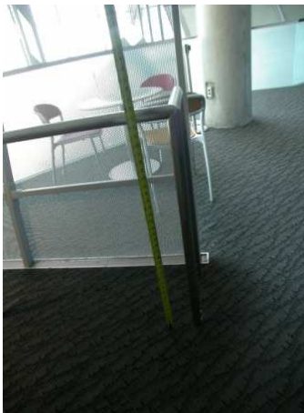
Figure 29 - Guardrail Not Cane Detectable on Level 3
