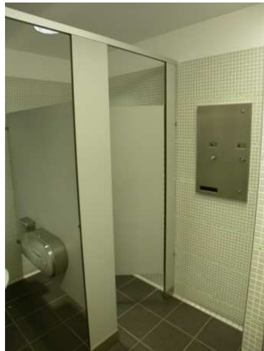
Figure 49 - Typical Inaccessible Feminine Napkin Dispenser
