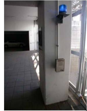
Figure 43 - Protruding Blue Lights
