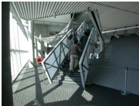
Figure 20 - Protruding Stair Railings
