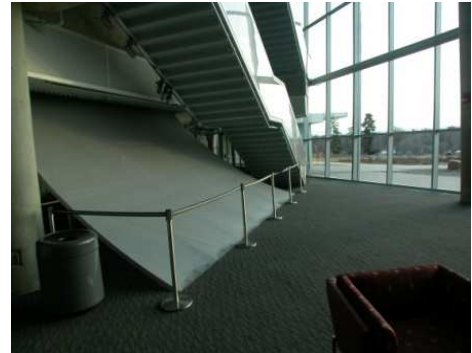
Figure 17 Tape Barriers Not Cane Detectable
