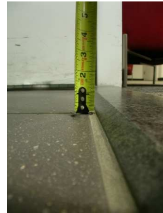
Figure 48 - Inaccessible Threshold at Typical Family Restroom Doors
