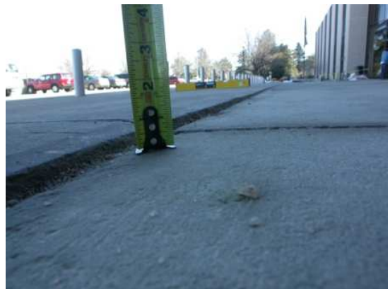
Figure 32 - Lip in Concrete at Main Entry Plaza
